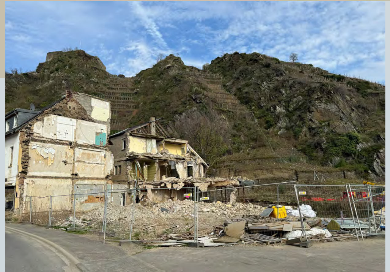
02 Mayschoß, devastating impact of the 2021 flood in the Ahr Valley
