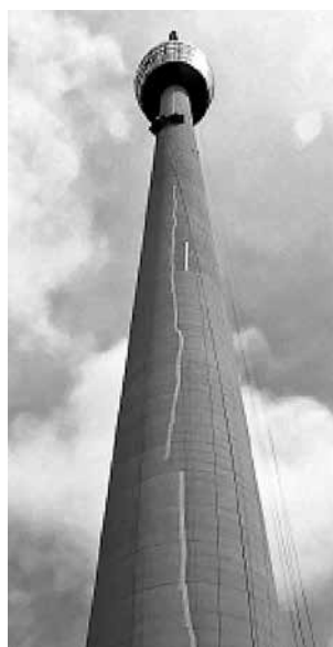
Fig. 6: Longitudinal cracks in the tower shaft
